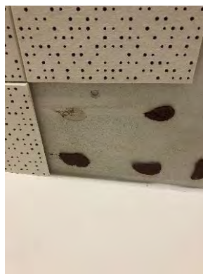
Ceiling tile mastic
